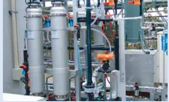
Groundwater purification system using GS modules
